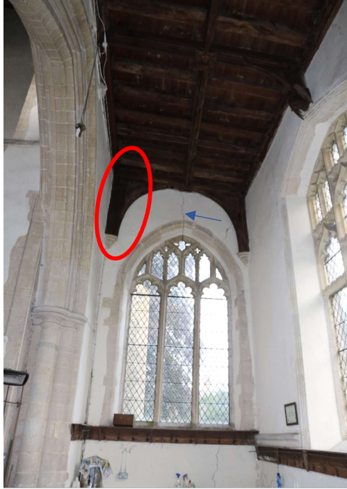
Figure 7. Western end of north aisle where droppings characteristic of Myotis (confirmed by DNA) were below a brace (red). Large masonry crack (blue).
