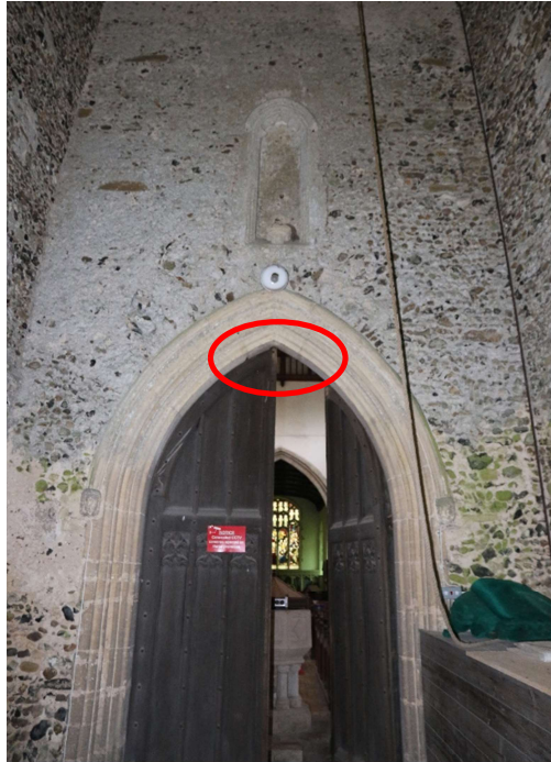
Figure 3. A gap around the frame of the tower door is used by bats as a primary access into the church.
