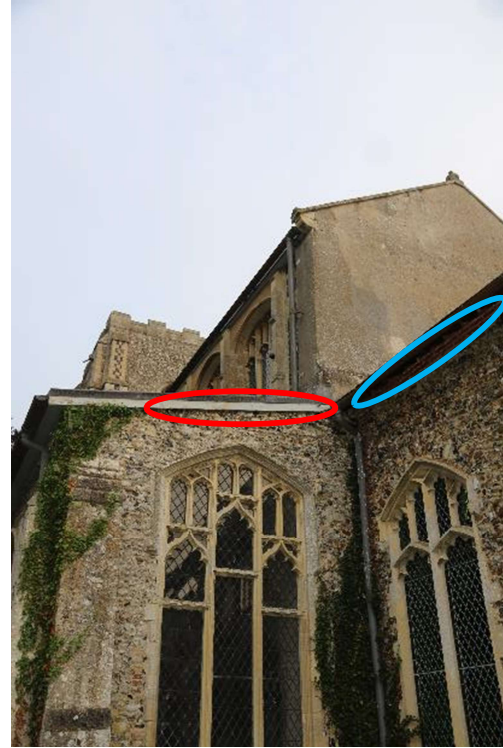
Figure 12. Fascia board (red) with gap behind on south aisle eastern wall and gaps under eaves (blue) of southern chancel wall.
