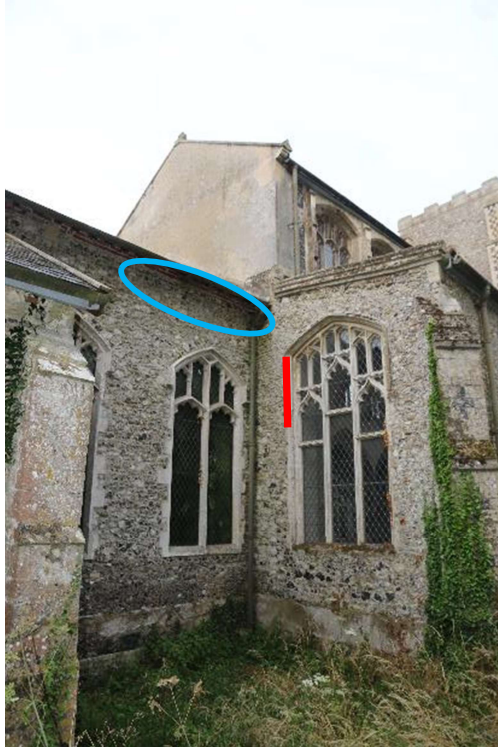
Figure 11. Gap (red) by the window on the eastern wall of north aisle and gaps (blue) under eaves of northern chancel wall.
