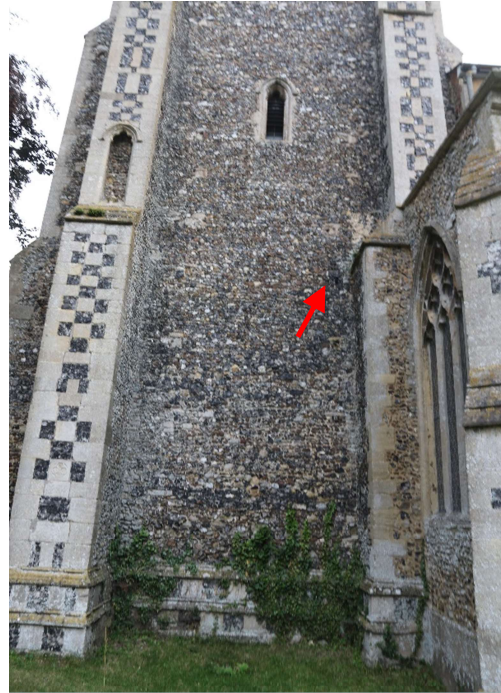
Figure 4. Tower with missing flints.
