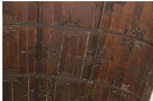
Figure 10. Decorative panelled ceiling with gaps which could allow bats into the church.
