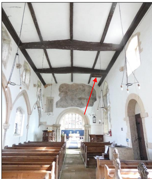
Photograph 3.2.7: The location of the hole in the nave ceiling is shown by the red arrow.
