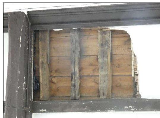
Photograph 3.2.8: Close-up view of the partially collapsed ceiling in the nave roof in the location shown by the red arrow in photograph 3.2.7. Bats that access the church interior predominantly do so via this hole in the ceiling. Many of these bats are then unable to return to the roost or exit the church via an alternative route.
