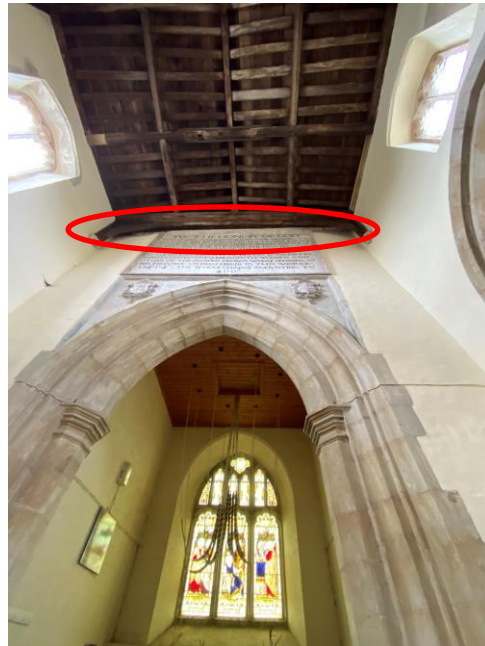
Photograph 5 Internal roosting areas between wall and timbers
