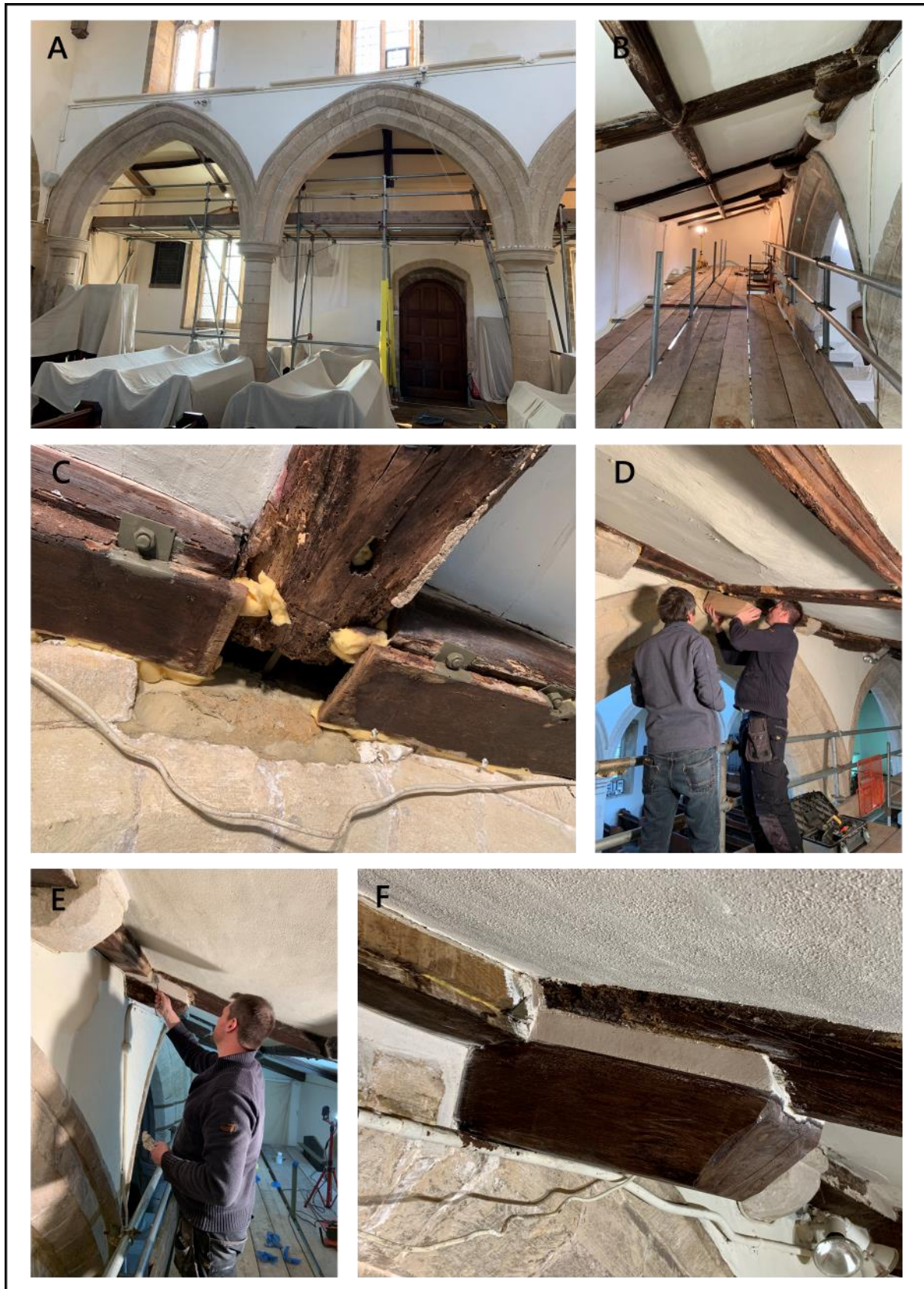
Figure 1. Photographs of works to block bat access from the roof roosts to the church interior (in 2018 temporary blocking with foam sponges, in 2019 made permanent with repair works to close-up bat access gaps in the south aisle).
