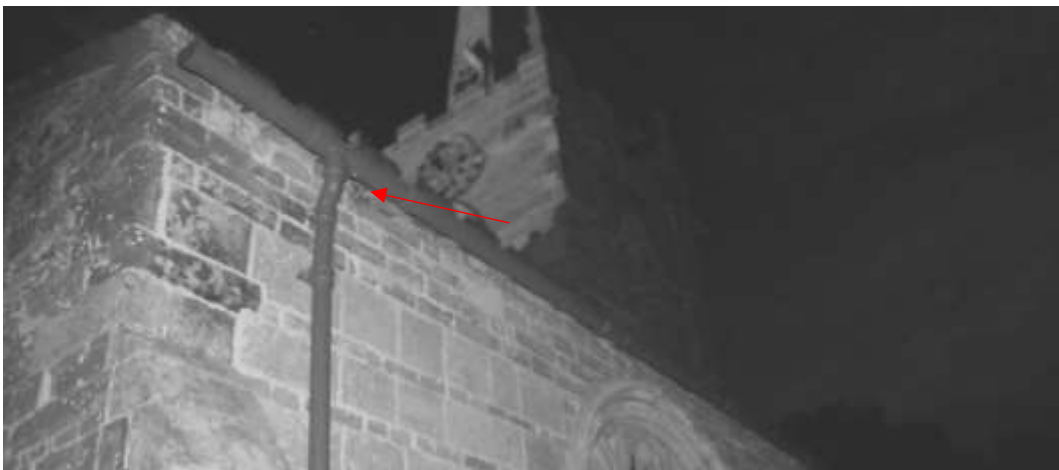
Photograph 3.1.9: The Natterer’s bats (re)enter the church via three gaps at the eaves of the north aisle. The red arrow shows the external location of one of these features - feature 4b, Figure 10.1.
