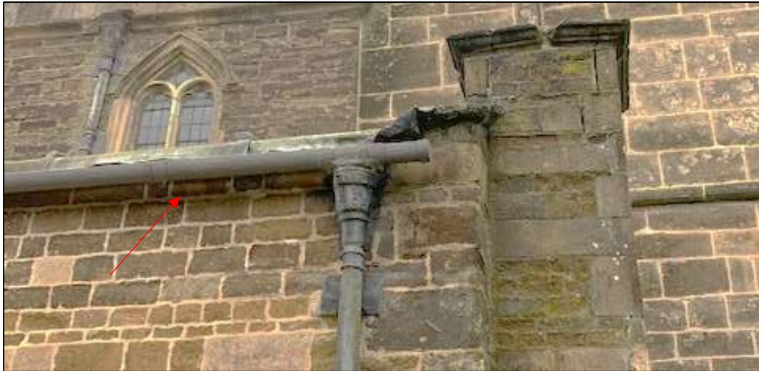
Photograph 3.1.8: The Natterer’s bats (re)enter the church via three gaps at the eaves of the north aisle. The red arrow shows the external location of one of these features – feature 4a, Figure 10.1.
