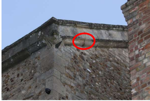
Figure 9. Cornice gap in the east nave wall.
