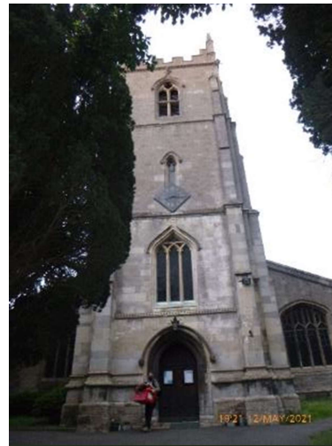
Figure 6. The western aspect of the church, showing tower, and north and south aisles.
