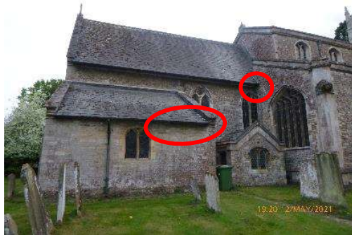
Figure 5. Northern aspect of the church, showing the roost access points in the north vestry and the chancel eaves.
