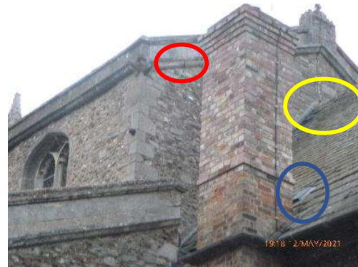
Figure 2. South eastern corner of the church, showing the raised roof tiles (yellow), possible Morris lead bat slate (blue) and a possible bat entry point in the cornice (red).
