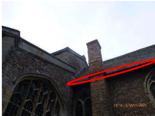
Figure 1. South eastern corner of the church eaves provide bat access points (red).
