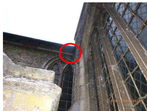
Figure 8. North eastern corner of the church provide roost access points (red).
