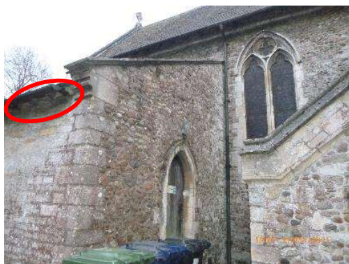
Figure 7. Walkway between the north vestry and the store. North vestry eaves provide roost access points (red).
