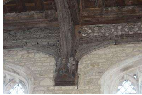
Figure 4. Closer view of the intricately carved truss end where pipistrelle have a primary roosting location.
