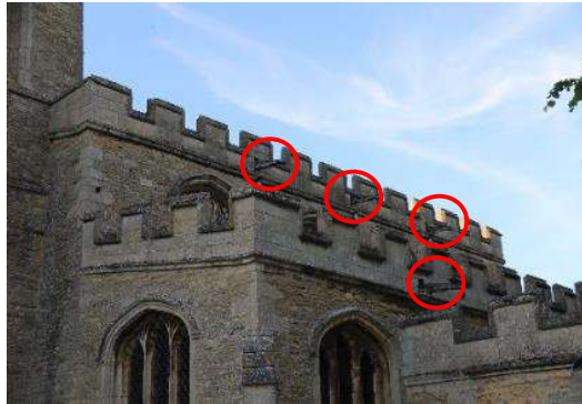
Figure 6. South aisle showing rainpouts from the nave roof and south aisle roof (highlighted).
