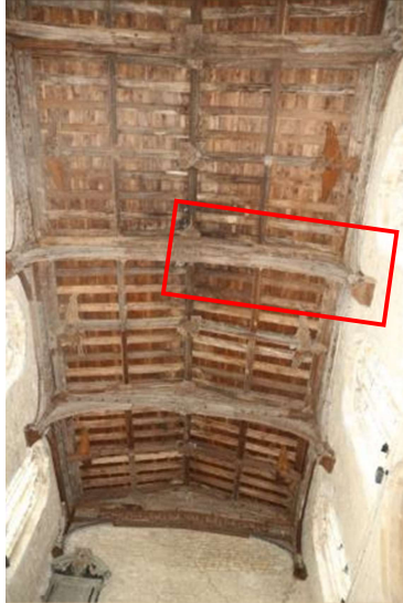
Figure 3. Internal view of the timber structure of the nave. The primary pipistrelle roosting location is highlighted (red).
