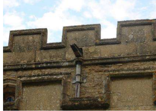
Figure 7. Rainpout from the nave roof where the primary pipistrelle roost access point is.
