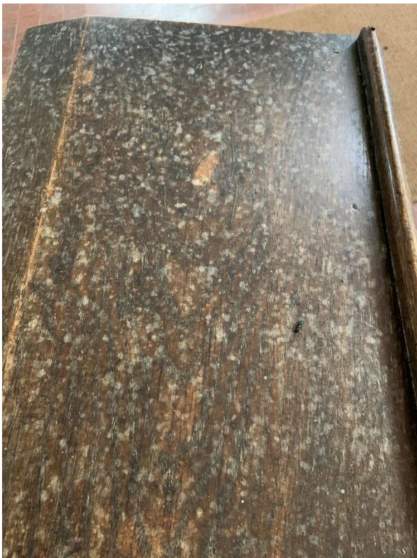
Photo 12. Urine staining to pews.
