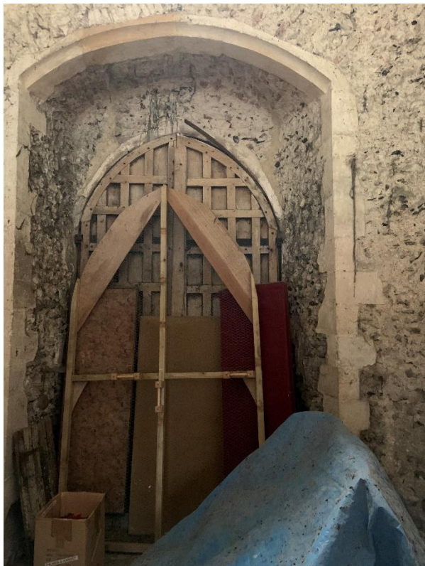
Photo 8. Tower/west door (main pipistrelle access, also used by Natterer's bats). Potential location for false doors to create an enclosed pipistrelle roost area between the two sets of doors (with the addition of a large, heated bat box).
