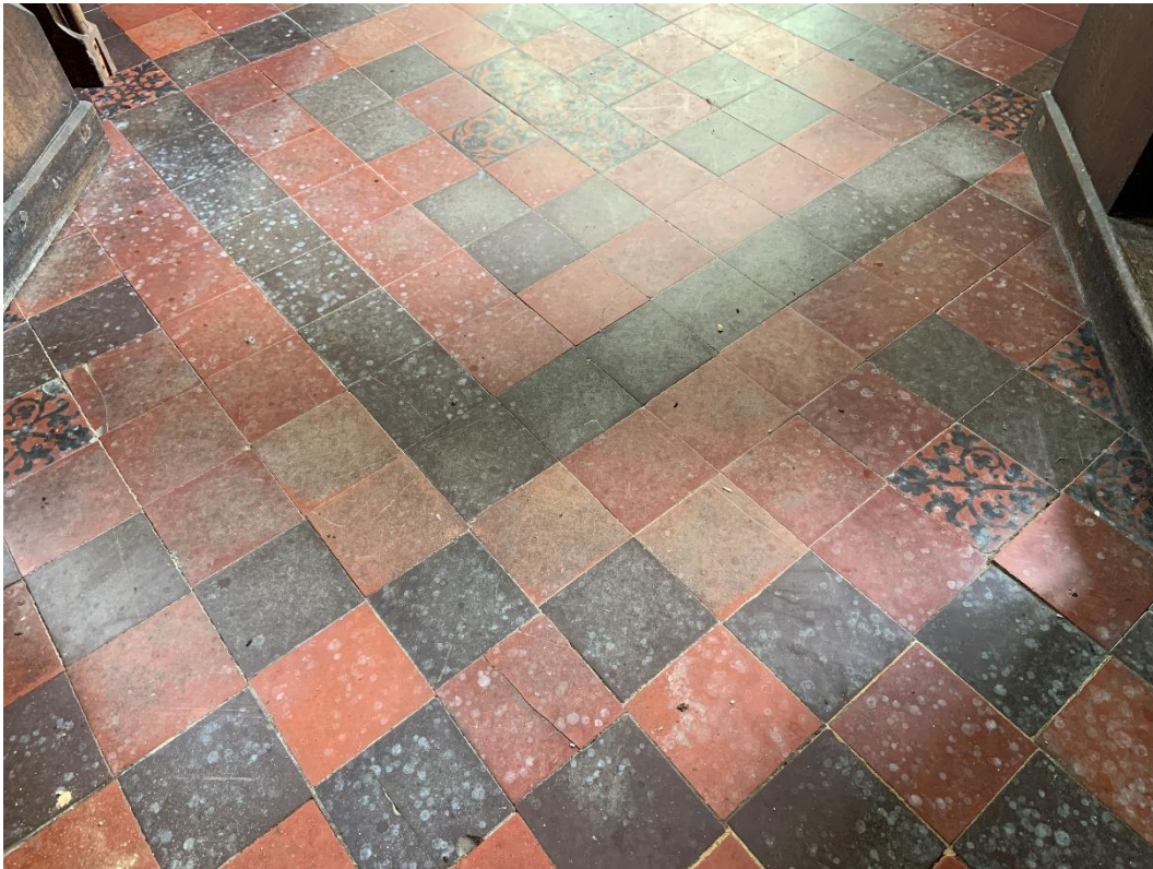
Photo 11. Urine bleaching to floor tiles.
