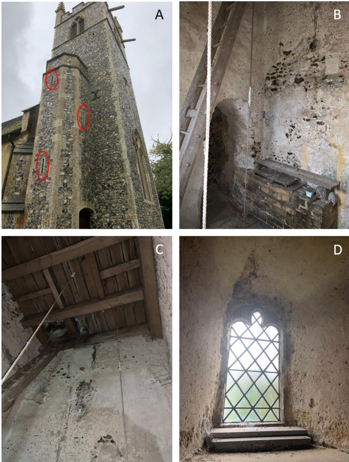
Figure 9. Photos of the tower, where roost enhancements are proposed. A. Tower exterior (entrance and first floor), potential bat access circled in red. B. First floor interior of tower (with doorway from stairway where slits are present, allowing bat access). C. First floor looking up to second floor (may be possible to fix bat boxes onto wooden floor structure). D. First floor window (will need covering on the inside to reduce light levels).
