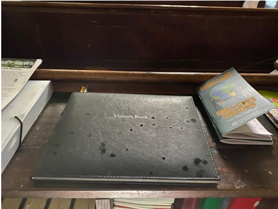
Photograph 3: Urine stains and droppings on internal shelf by front porch
