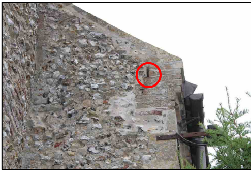
Figure 10 – West end of the nave by the tower showing the bat access slot A, installed as part of the 2012/13 works. The bat box in figure 3 is immediately behind this slot. A peak of 508 soprano pipistrelles emerged from this slot on the bat night in August 2019
