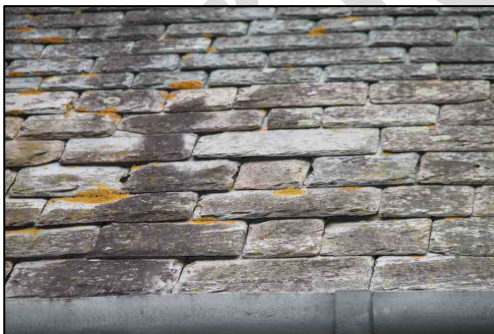
Figure 12 – Gaps under slates on the chancel providing potential bat roosting areas for individual bats (only the nave was re-roofed in 2012)
