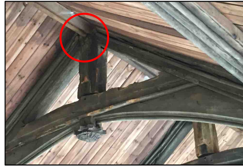
Figure 15 – Detail of the principal rafter above which the common pipistrelle maternity roost previously roosted. However, this location is now only used by the occasional bat
