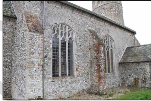
Figure 11 – Eaves detail and brick buttresses on the north side of the nave
