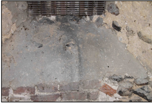
Figure 20 – Droppings on the windowsill within the silence chamber. Bats are able to access around the mesh
