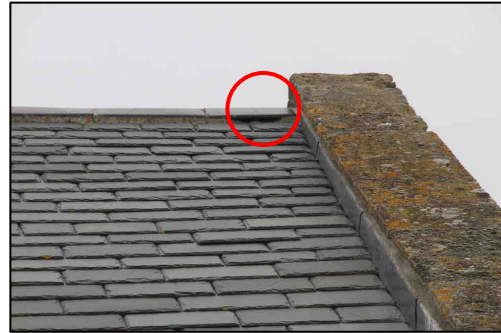
Figure 9 – Nave ridge showing bat slot B installed as part of the re-roofing works in 2012/13 to replace lost roosting areas in the roof structure. A peak number of 57 common pipistrelles emerged from this location in June 2019
