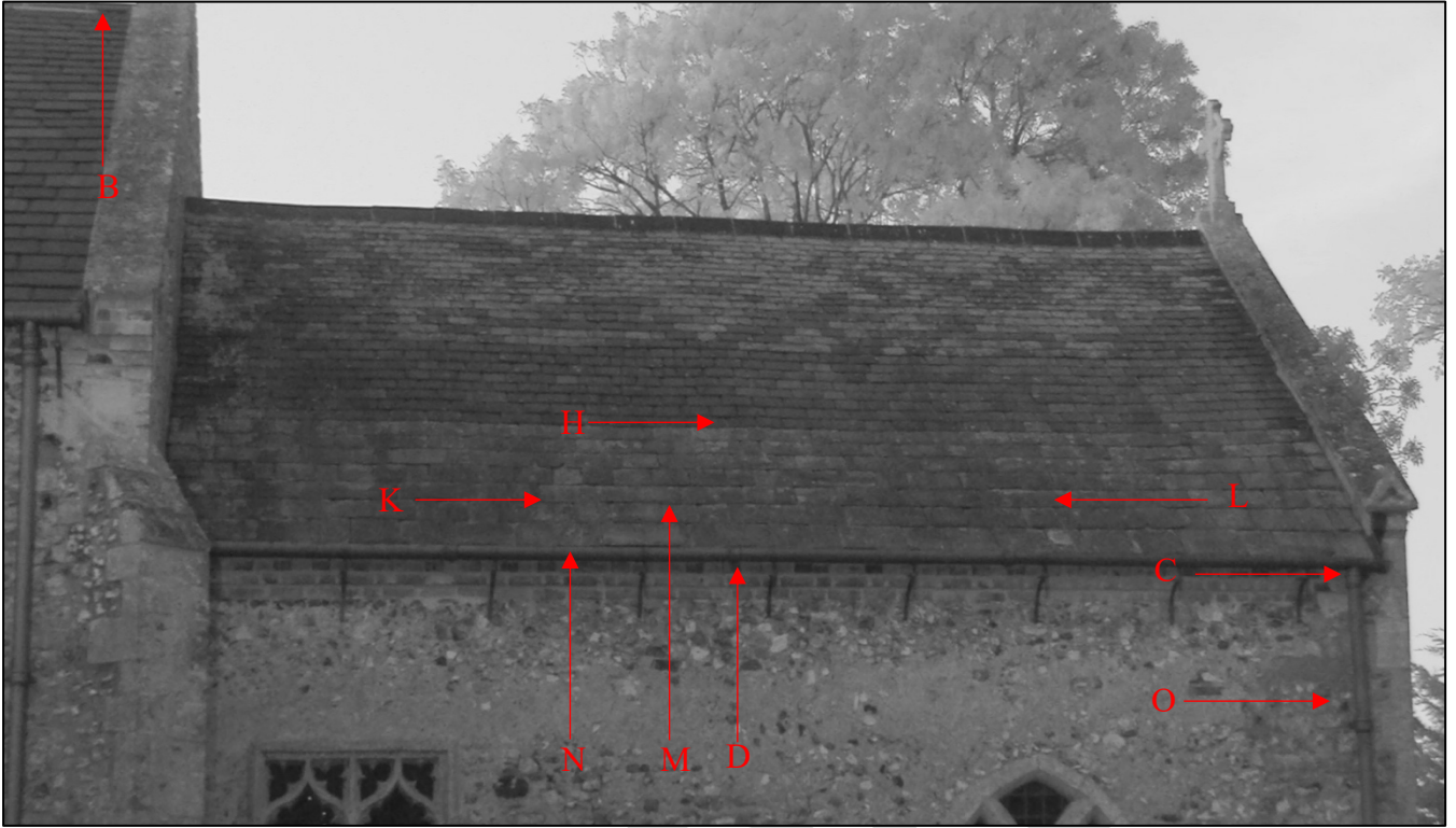
Figure 26 – Bat roosting locations on the southern elevation of the chancel and west end of the nave
