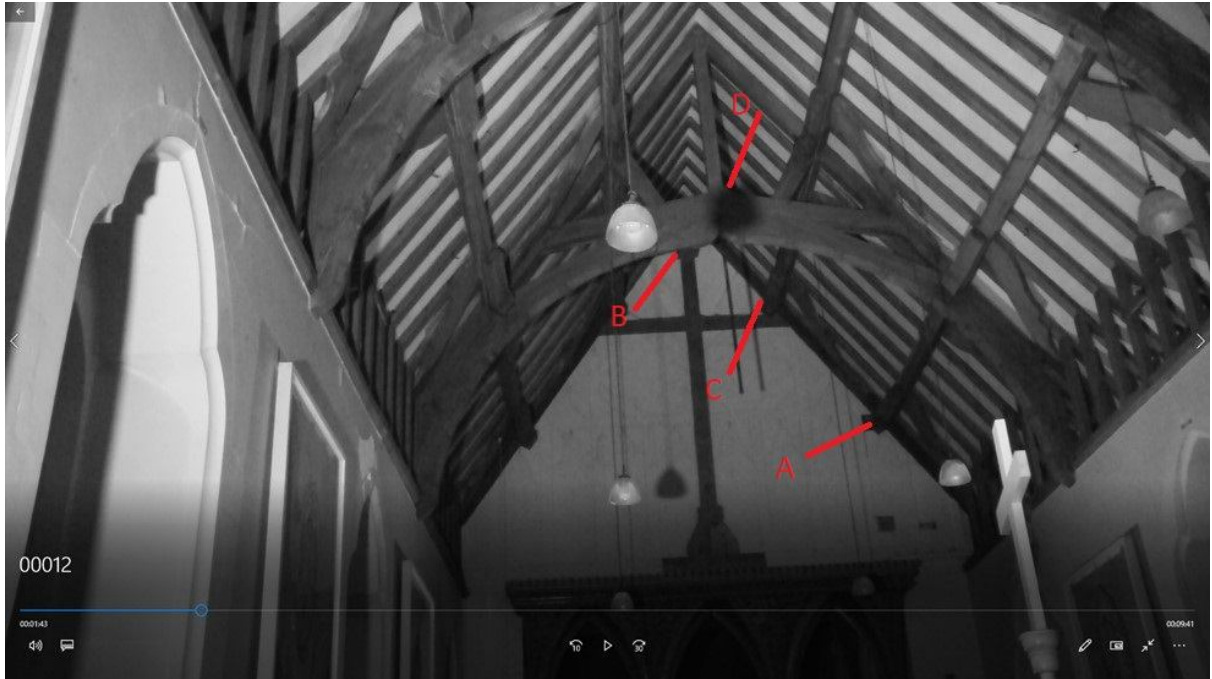
Brown long-eared bat internal roosting points, east end of nave. Number of bats emerging from each point: A-10, B-1, C-4, D-1.
