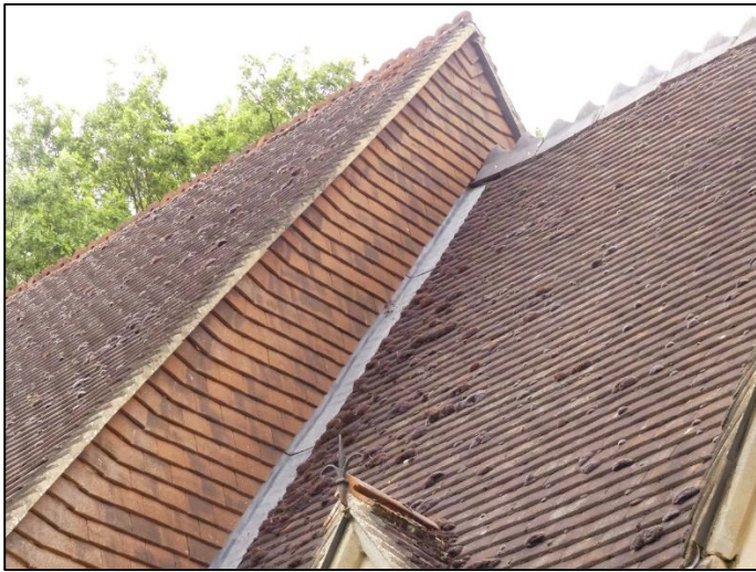
Close-up of hanging tiles on east end of nave gable. Note gap below the chancel apex, adjacent to the hanging tiles.
