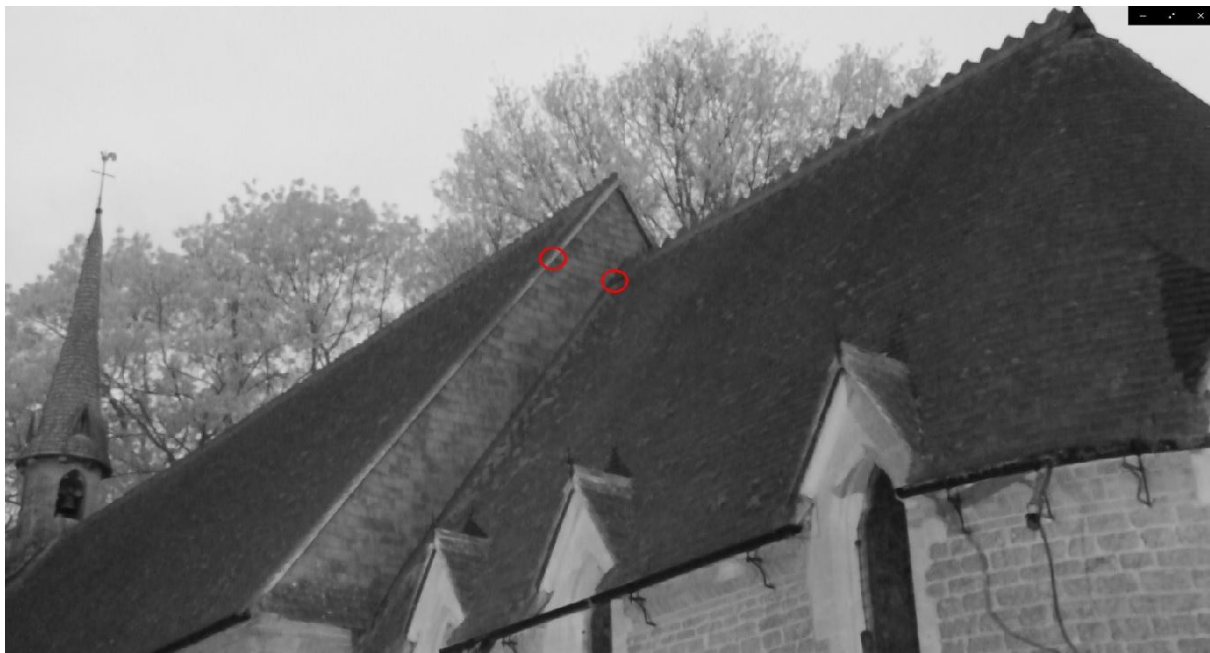
Emergence points of one soprano pipistrelle (left circle) and two brown long-eared bats (right circle).
