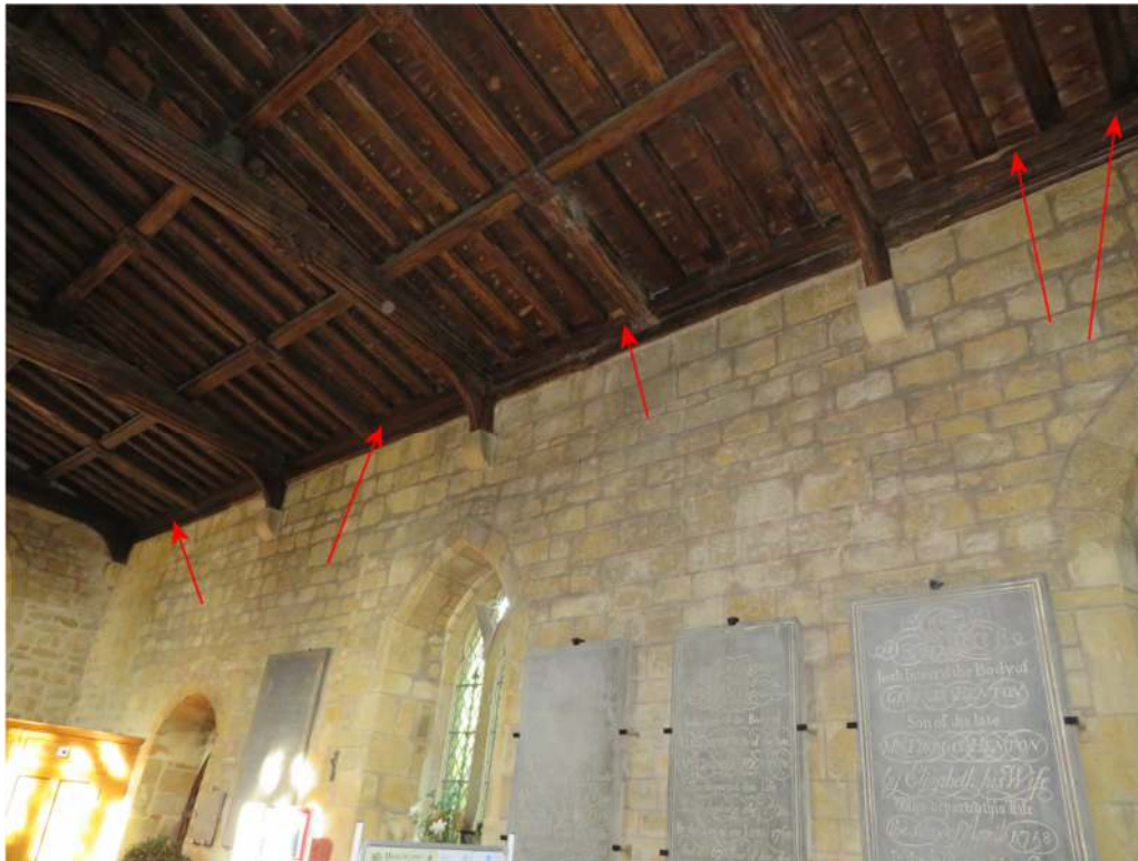
Photograph 17. Location of bat egress points at the top of the north wall of the north aisle (excluding access points at the corners)
