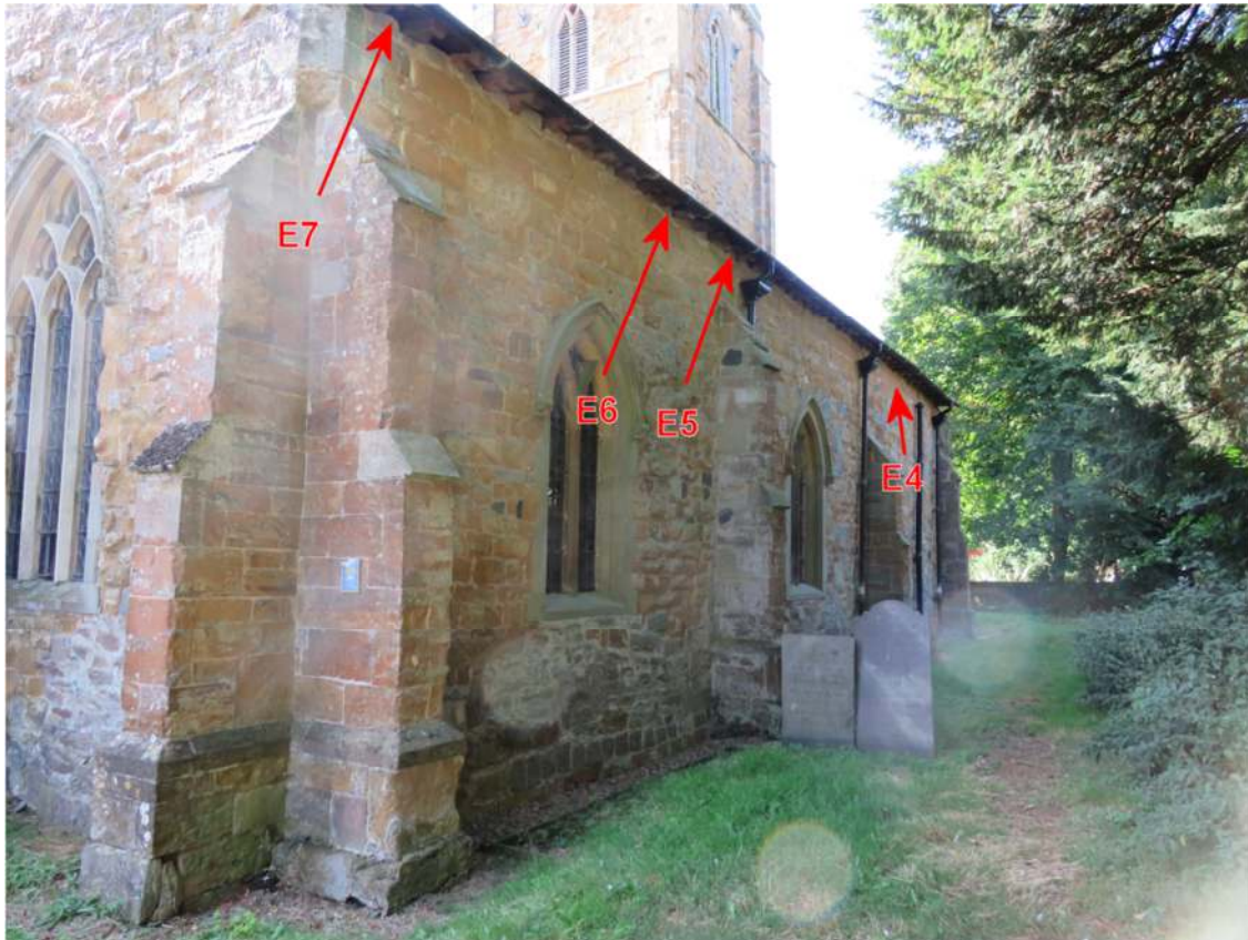
Photograph 11. Location of bat access points along the north wall of the aisle (view from north-east corner)
