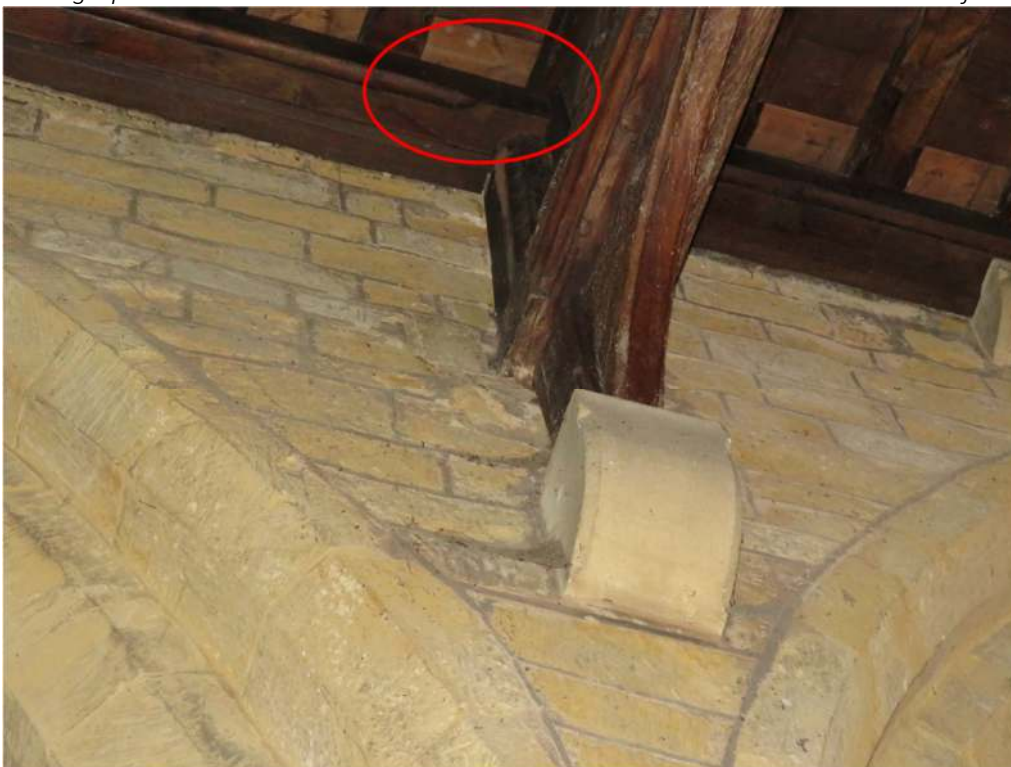
Photograph 21. Daubenton's bat roost behind the truss at the top of the first pillar from the eastern end of the north aisle
