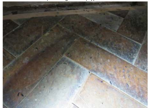
Photograph 9. Pipistrelle bat droppings at the south-east corner of the south aisle (see Figure 2 (g))
