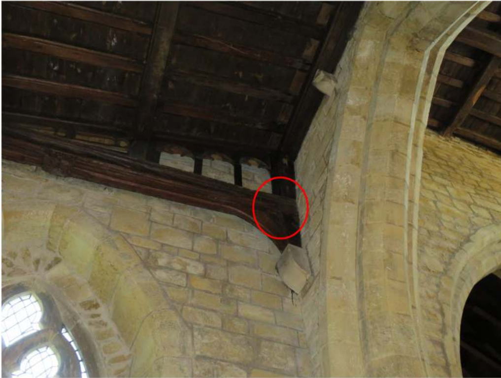
Photograph 18. Main Daubenton's bat roost behind the truss at the south-east corner of the north aisle
