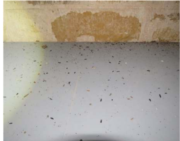
Photograph 5. Daubenton's bat droppings on top of the toilet at the north-west corner of the north aisle (see Figure 2 (c))
