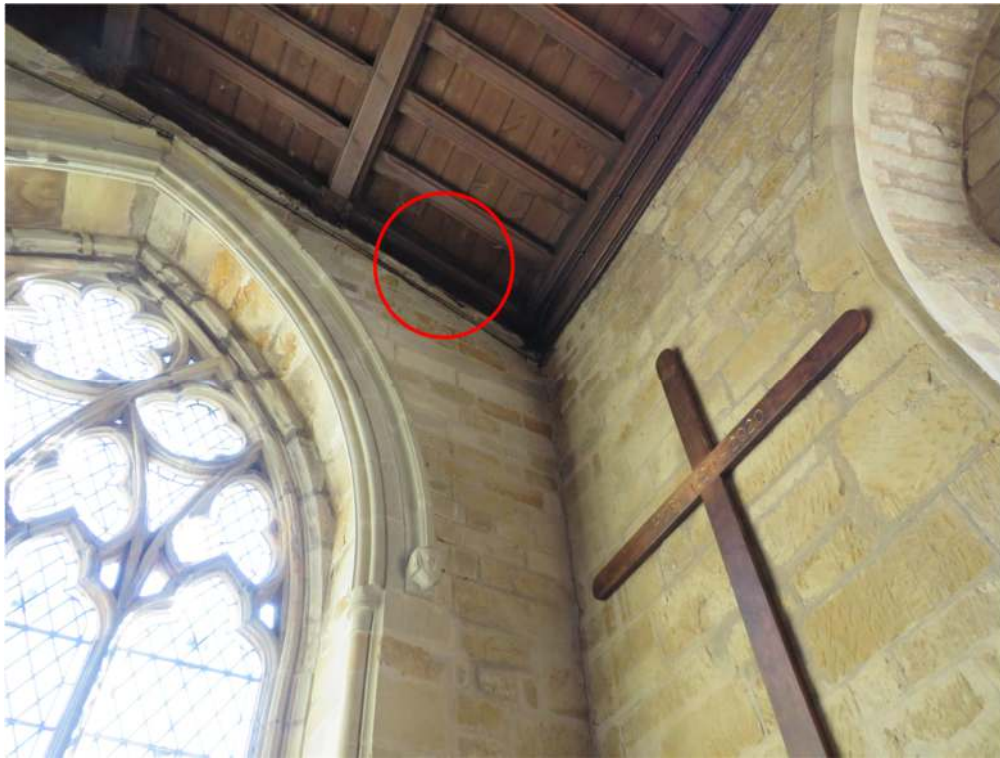
Photograph 24. Common pipistrelle day roost behind the end rafter at the south-east corner of the south aisle
