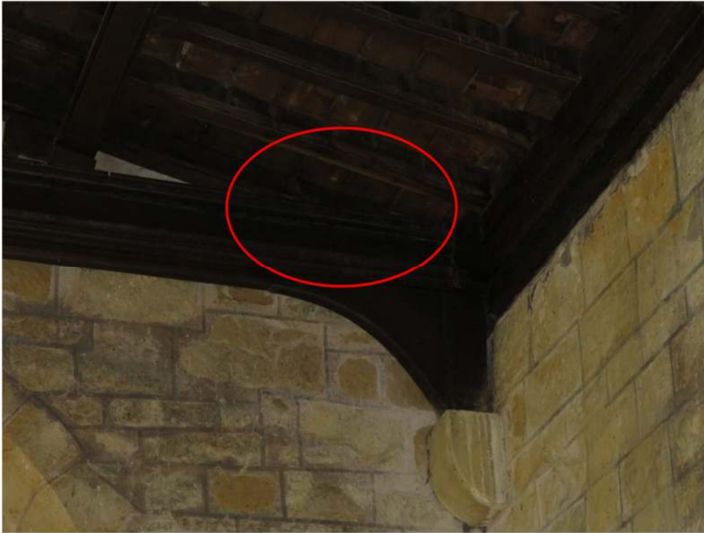
Photograph 20. Daubenton's bat roost behind the truss at the north-west corner of the north aisle
