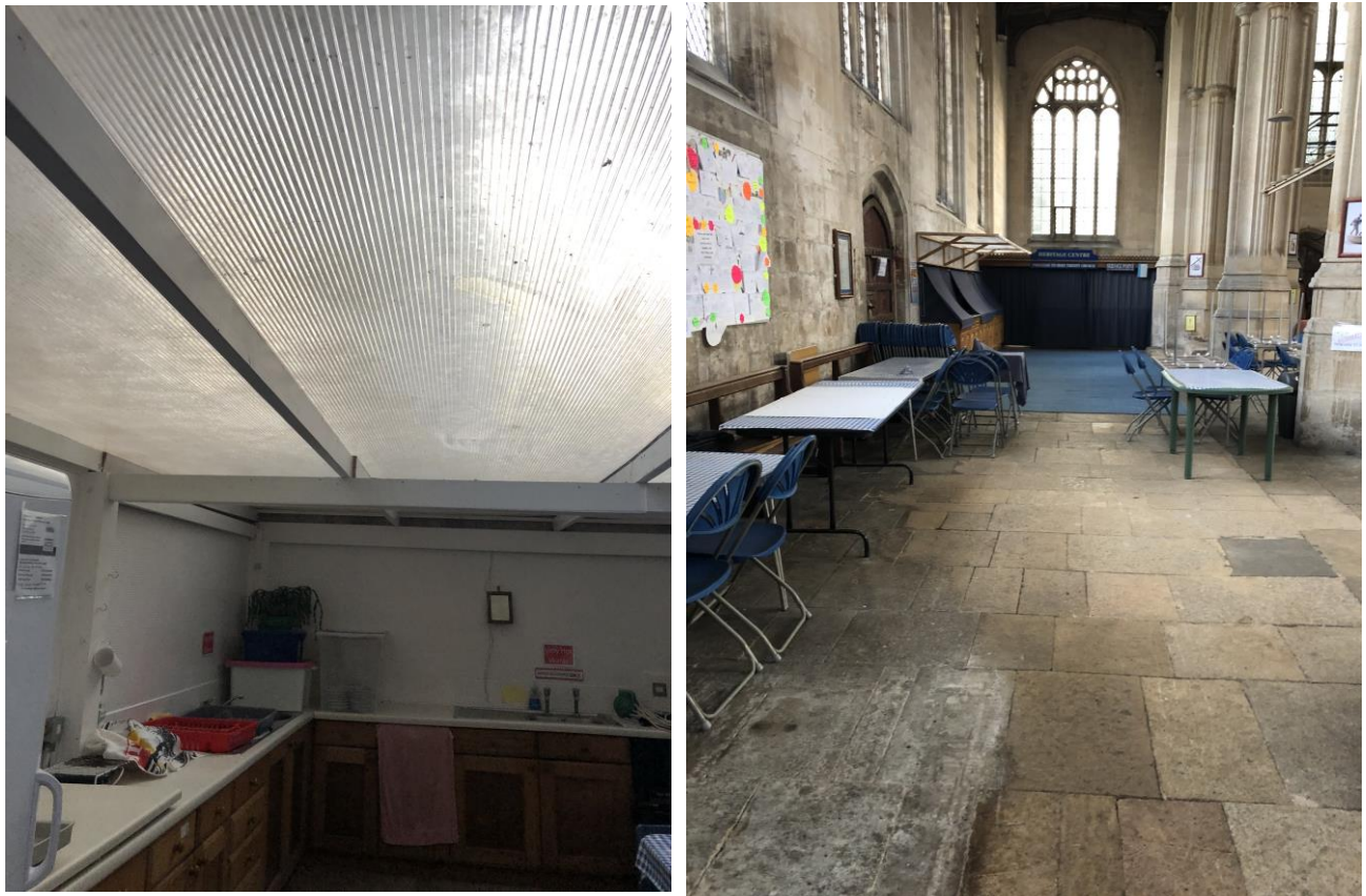
Photograph 3 - showing the lack of droppings on the roof of the Heritage Centre and on the floor of the South aisle
