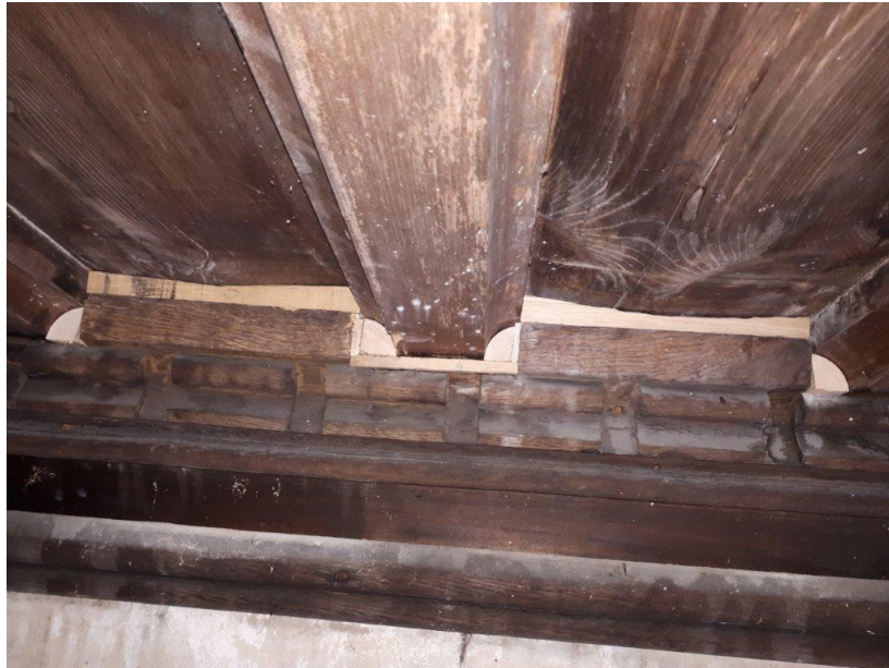
Photograph 2 - showing the gaps following infilling by the contractors' joiners
