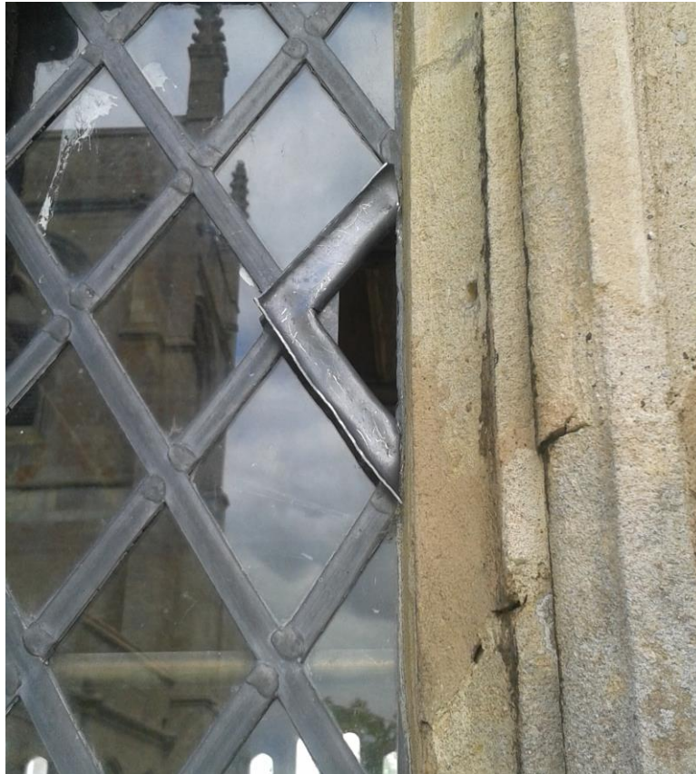
Photograph 5 - showing the new bat access point which was installed in the high-level windows on the Western south of the south transept
