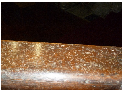
Photo 4 Urine damage to wooden hand rail
