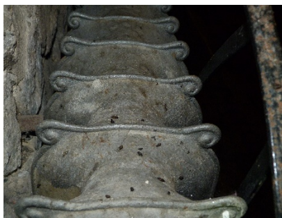
Photo 6 Droppings on radiator
