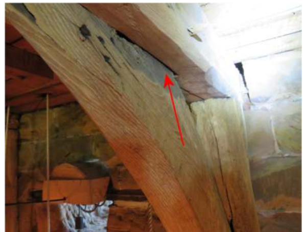
Photograph 5. Crevice in the tenon and mortise joint above the droppings shown in Photograph 4
