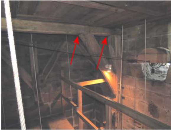
Photograph 6. Crevices in tenon and mortise joints above bat droppings in the silence/clock chamber
