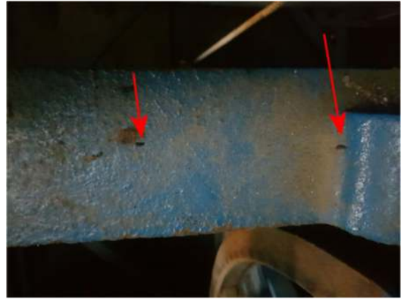
Photograph 7. Example of bat droppings on the metal frame supporting the bells
