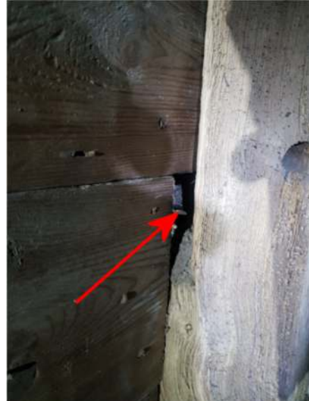
Photograph 3. Opening between the timber frame and the wall above the droppings shown in Photograph 2.
