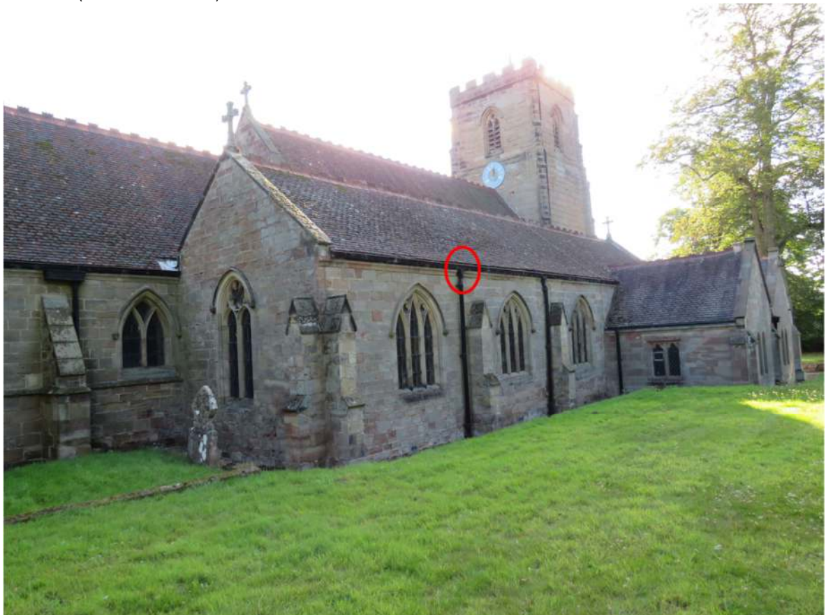
Photograph 19. Access point at top of drainpipe on the northern side of the church (see Photograph 18)
