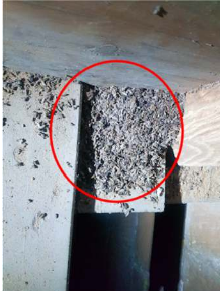
Photograph 2. Large accumulation of bat dropping to the right of the clock mechanism in the north-west corner of the silence/clock chamber
