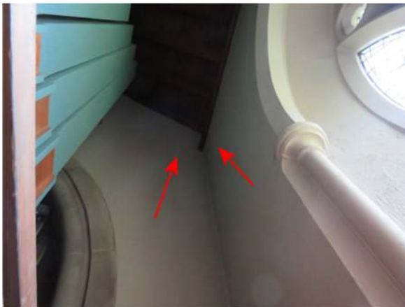
Photograph 10. Bat droppings adhered to the walls at the north-west corner of the vestry/organ room
