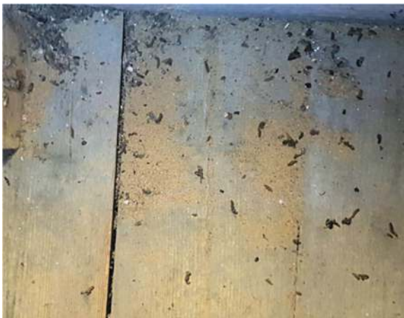
Photograph 4. Accumulation of droppings on the floor at the south-east corner of the silence/clock chamber
