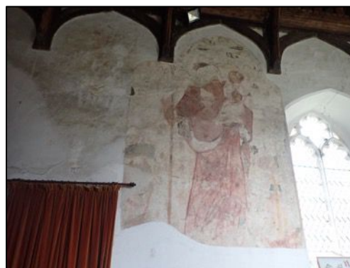
Figure 16 – Wall painting in the north-west corner of the church, close to the principal access A1. Some bat droppings were present on the wall painting, but most were aged when inspected from scaffolding with Dr Andrew Kerkham on the 13 th August 2019
