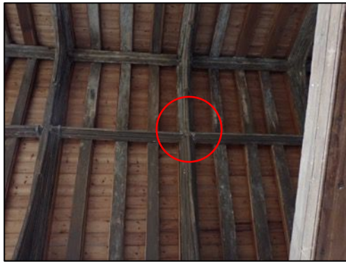
Figure 21 – Roof structure with the roosting area where the common pipistrelle roost was present in June 2014
