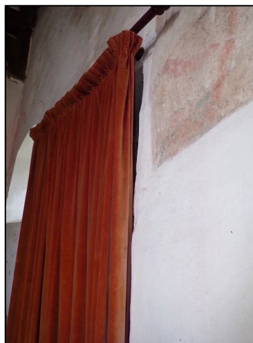
Figure 18 – Curtain over the north door over which the serotina and a common pipistrelle exited in June 2019 (A2)
