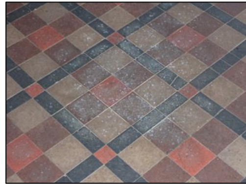
Figure 22 – Old urine staining on the chancel tiles below the previously identified main roost site 2014
