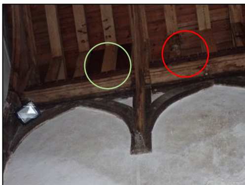
Figure 17 –Bat boxes on the north-western elevation (green) and principle access area (red) A1
