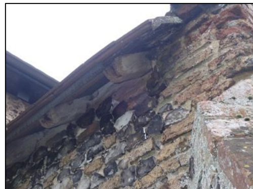
Figure 12 – Detail of porch eaves roosting location A3 for up to 2 common pipistrelles
