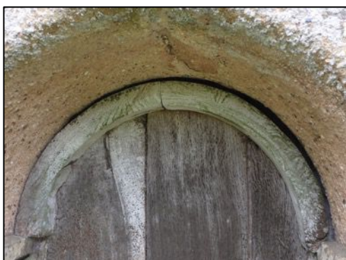
Figure 19 – North door access (externally) showing gap over
