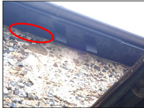
Figure 10 – South nave soffit, previous access point noted to the west in red
