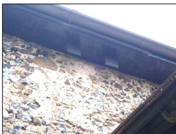
Figure 3 – 2 of the bat boxes that were installed during the roof repair works in 2015 (south side of the church)
