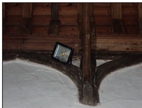
Figure 20 – One of many internal eaves details which have bat roosting potential via open joints and cavities
