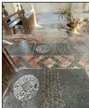
Figure 21 – Ledger stones in the nave of high significance. These show a high level of historic and current bat urine damage. These are shown close to roost R3 and therefore suffers significant damage
