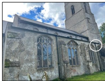
Figure 15 – North aisle and nave, showing the location of principal natterer's access point A1
