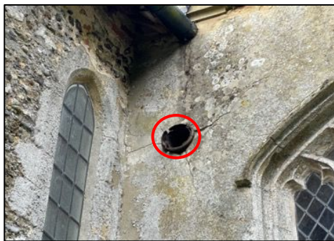
Figure 27 – Location of flue pipe on the west side of the north aisle
