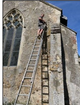
Figure 7 – Installation of the additional putlog holes on the east face of the chancel
