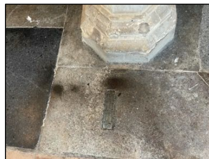
Figure 11 – Droppings and debris below roost site R2 in the south aisle
