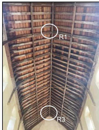
Figure 8 - The nave roof structure provides a multitude of roosting opportunities including principal areas roost R1 and R3
