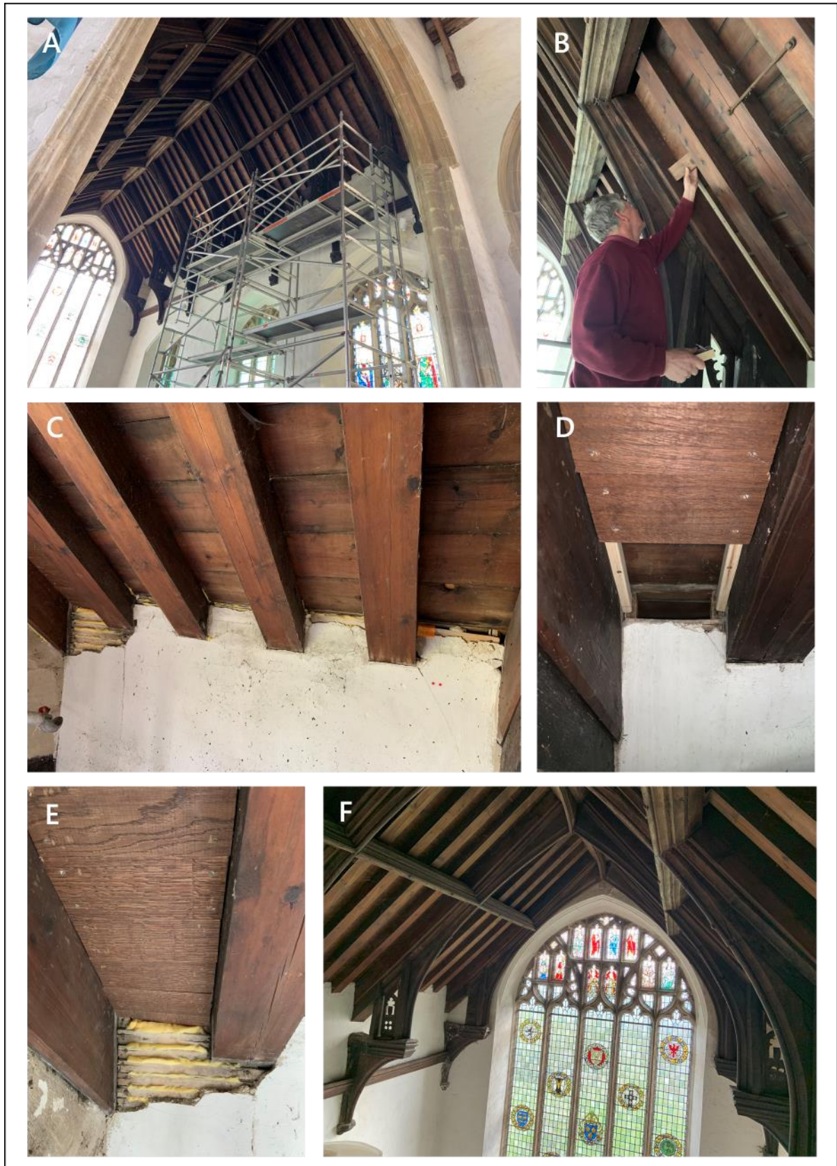
Figure 1. Photographs of interior works (chancel) – rafter bat boxes (south side) and blocking of gaps in plasterwork through to eaves roof void.
