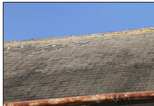
Figure 11 – Loose and missing slates on nave giving potential bat roosting area although no bats were seen to emerge
