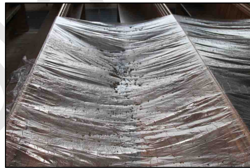
Figure 15 – Droppings on sheeting on the pews under the main roost area
