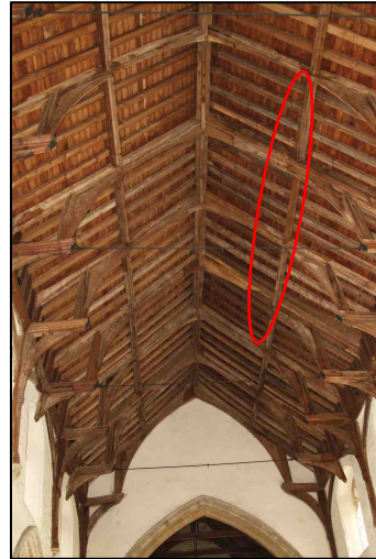
Figure 13 – Nave roof where most bat roosting takes places, typical locations are at the junctions of the purlins/rafters on the south side and above the ridge
