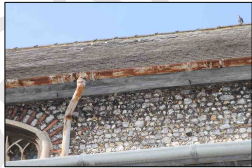
Figure 9 – Eaves detail on the south side of the nave showing the soffit with gaps. Again, no bats were seen to emerge from these locations during the surveys
