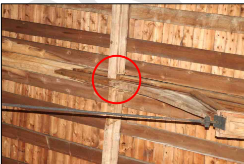
Figure 16 – One roost location by a purlin on the south side of the nave
