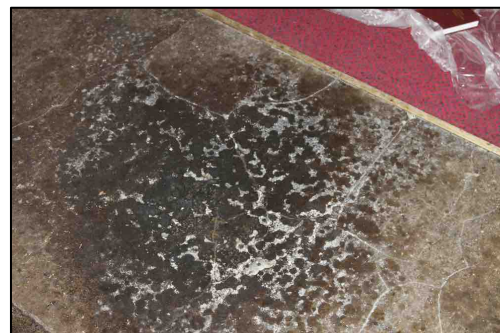
Figure 17 – Urine staining eroding limestone floor slabs
