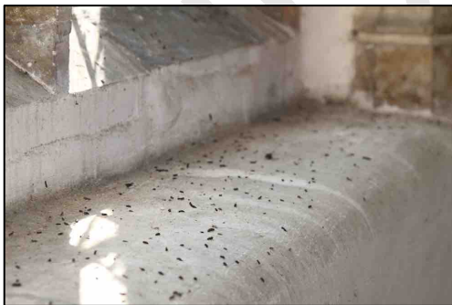
Figure 22 – Droppings on windowsill in the north aisle
