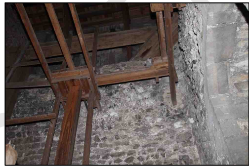
Figure 27 – General view of the bell chamber. A potential number of roosting areas but no evidence noted
