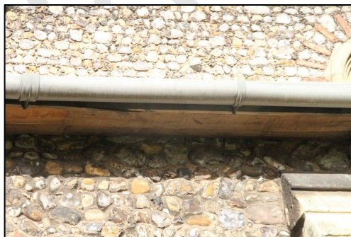
Figure 30 – Timber boards under rafters on the south aisle. These were put in as part of the works to the south aisle to try and provide alternative external roost areas. There was no evidence of any bat access during the 2019 surveys
