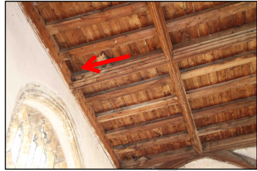
Figure 25 – Roof structure close to the access in the south aisle, south access point
