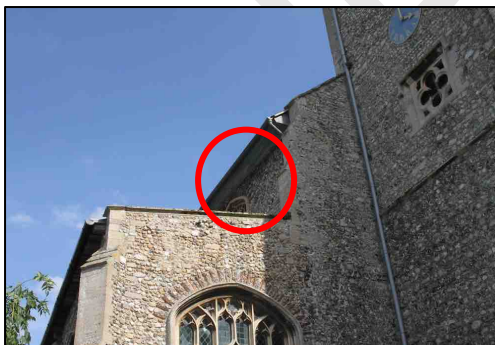
Figure 10 – Principal access from the church via the north-west clerestory window, viewed from the north side of the tower
