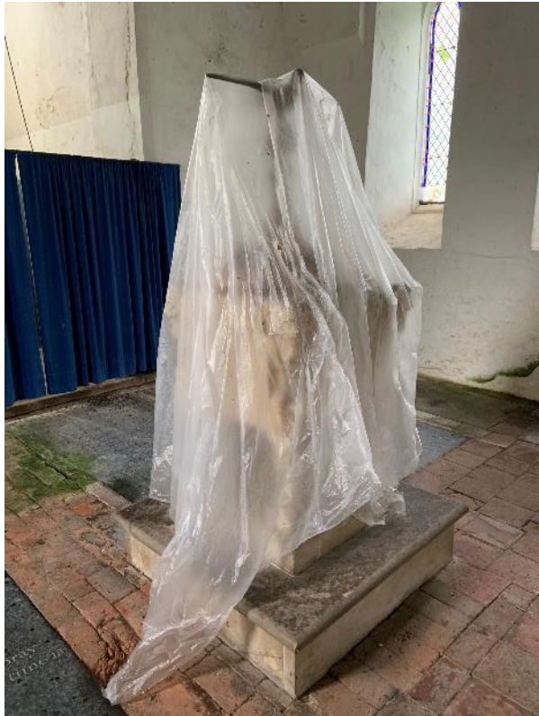
Photo 13. Font covered with plastic sheeting for protection from bat droppings/urine.
