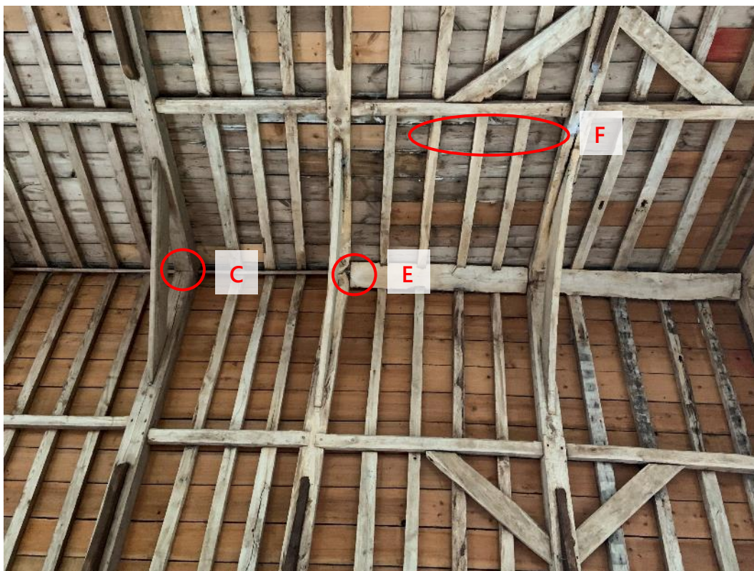
Photo 8. Nave roof interior (west end), roosts circled in red and labelled (see Figure 7). C is a common pipistrelle roost, E & F are Natterer's bat roosts.
