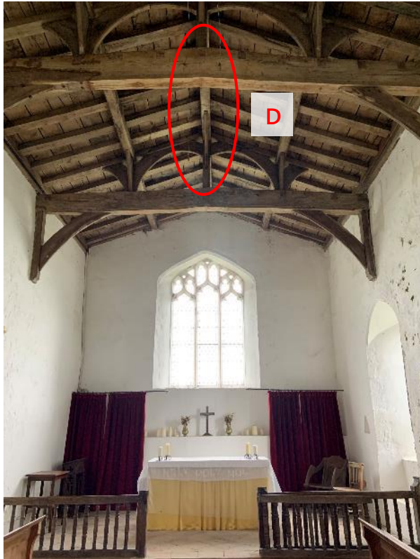
Photo 5. Chancel interior (facing east). Probable common pipistrelle roost above central ridge beam/sarking boards circled in red (roost D in Figure 7).
