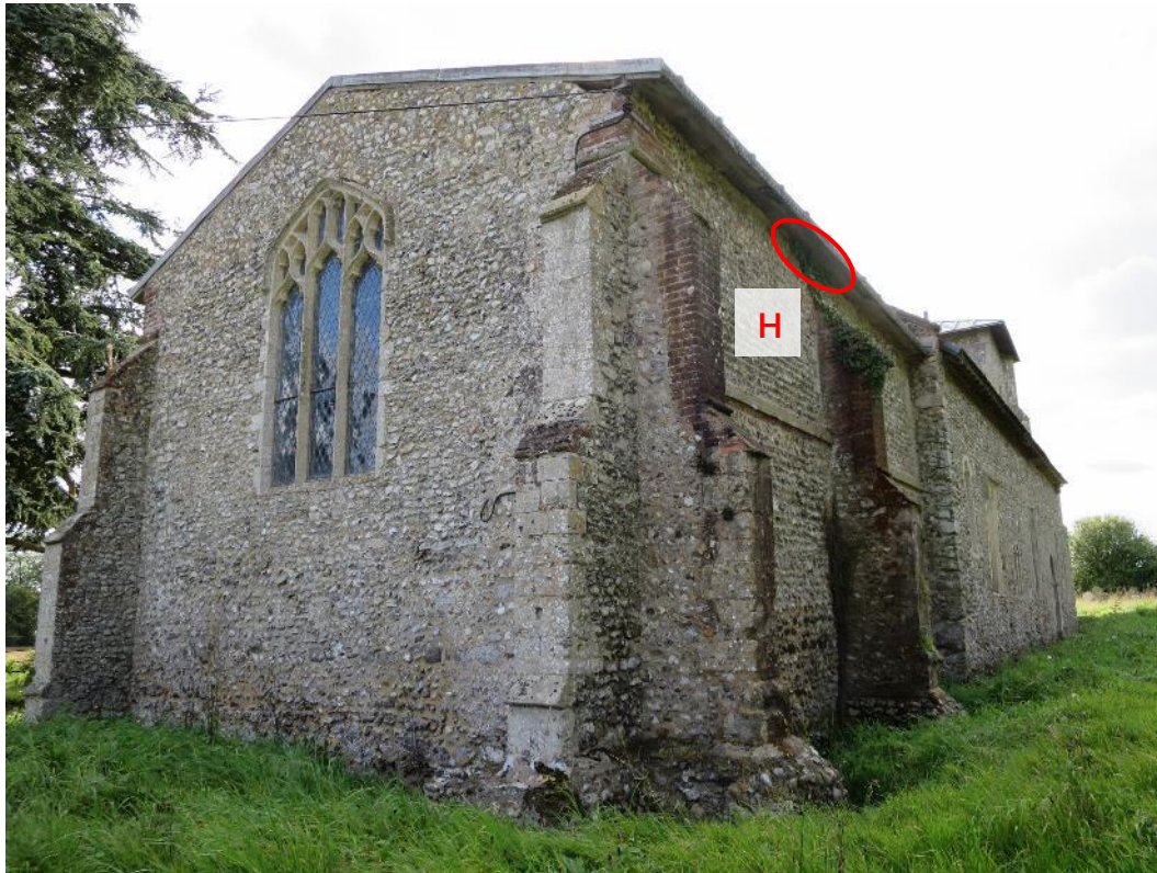
Photo 3. North-eastern end of chancel, with 'exterior' common pipistrelle roost area circled in red (access at eaves, around ivy patch, roost H in Figure 7).
