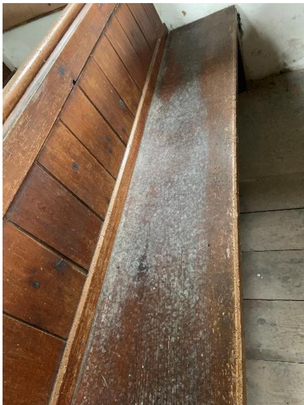
Photo 14. Bat urine bleaching on pews.
