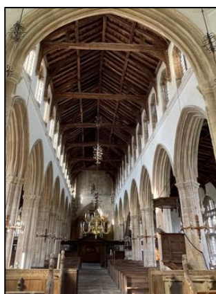
Figure 11 - The nave roof is of high significance. It is difficult to tell what impacts the bats are having due to the scale
