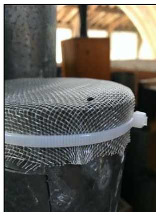
Figure 26 – Detail of the gauze with dropping on the top
