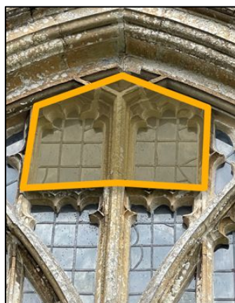
Figure 28 – Heated purpose-built bat box above north-eastern north aisle window. Ideally, this would go in the inside of the window so the bats can access via the existing tracery
