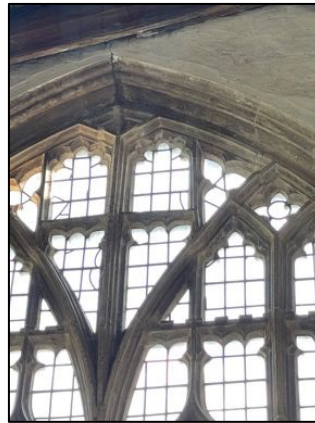
Figure 8 – Primary access A1 via the north- east north aisle window. The painting below the access suffers some damage from bat droppings and urine.
