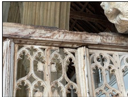
Figure 17 – Damage to the top of the screen in the north aisle. This is close to R3. This appears to be death watch beetle damage but the presence of bat urine which could enhance humid conditions for death watch is notable.
