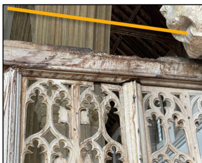
Figure 23 – Location of deflector board, possibly hung by chains over the rood screen
