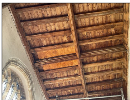
Figure 32 – An example of a rafter box at Thornham Church. Initially this is left open but after a year it will be connected to the access at the eaves
