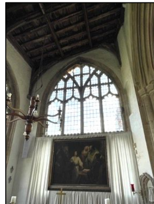
Figure 22 – Location of painting below bat access R3 has bat droppings on it due to the access above
