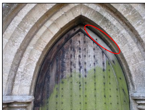
Figure 14 – Outside of the north door showing where the lichen has been worn away, presumably by the bats landing on the door.
