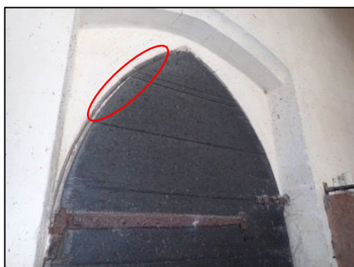
Figure 13 – Large numbers of droppings on the north door indicating the principal access point into the church. The main area for access is highlighted red.
