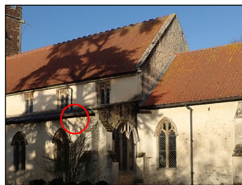
Figure 10 – Location of occasional pipistrelle access/roost E on the south side of the nave
